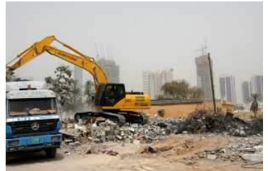
Demolition work has begun in the Satwa neighbourhood of Dubai for Jumeirah Garden City, but Meraas has not yet specified which of three building plans it will pursue. Pawan Singh / The National
