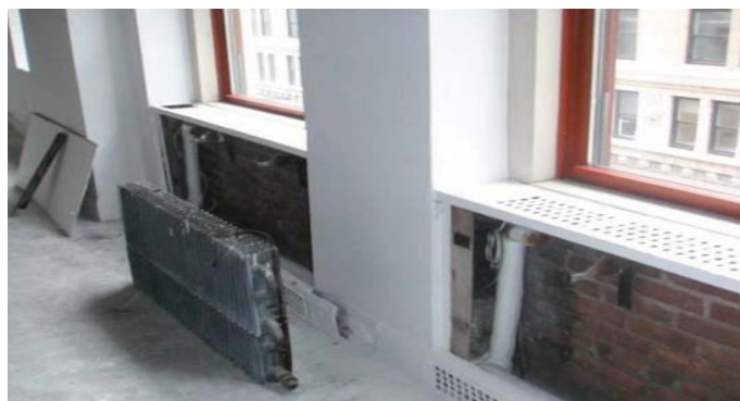
Installing insulated reflective barriers behind radiator units on the perimeter of the Empire State building
